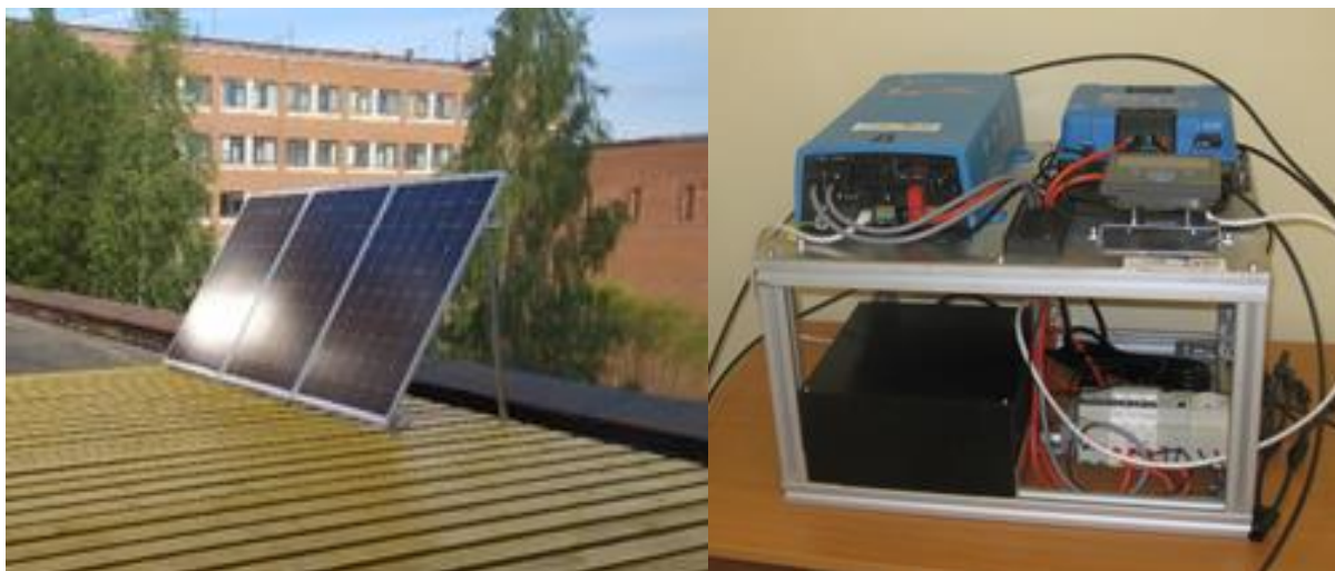
Fig. 1. Experimental solar electric generating station
